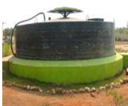
Fig. 4 Gas Storage Tank
