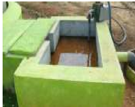
Fig. 5 Slurry Collection Tank
