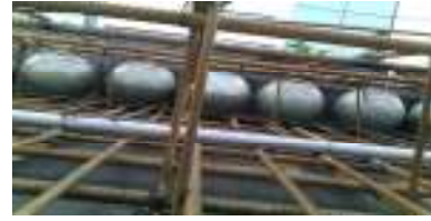
Fig 2: Bubble Deck slab a). Concrete grid frame set; b) slab installed with bubbles; c) c/s view of bubble deck slab
